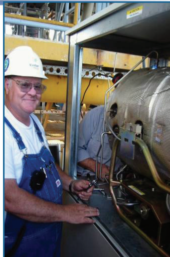
Servicing injectors at 20,000 hrs on a BP platform Capstone MicroTurbine
