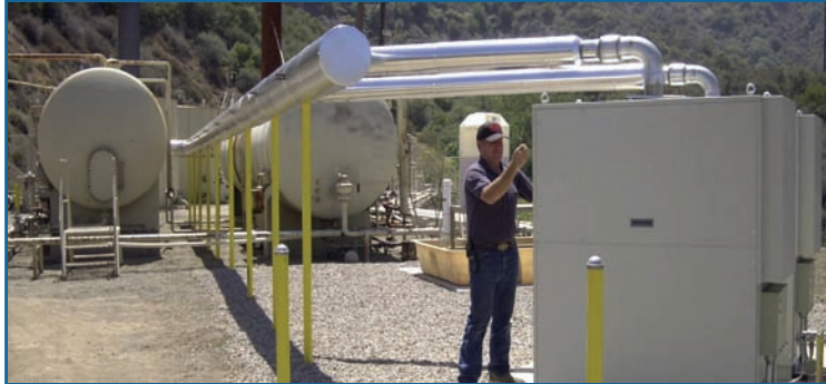
Heat from two C30s running on untreated wellhead gas goes to "heater/treater" separator
