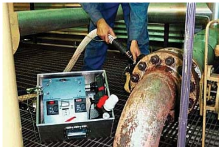
Leak Measurement Using a High Volume Sampler
