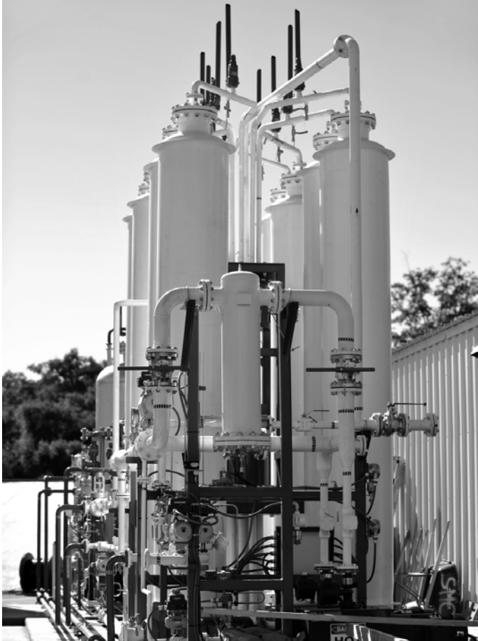
Xebec Pressure Swing Absorption Unit at the HARRF
