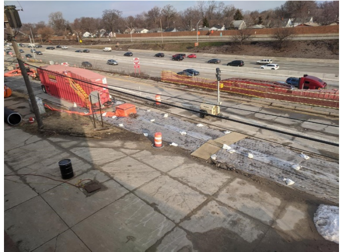
Photo of completed interceptor trench and frac tank along the service drive.
