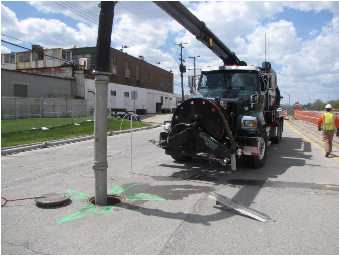
Vacuum truck with high pressure pump cleaning out the storm sewer line along the service drive.
