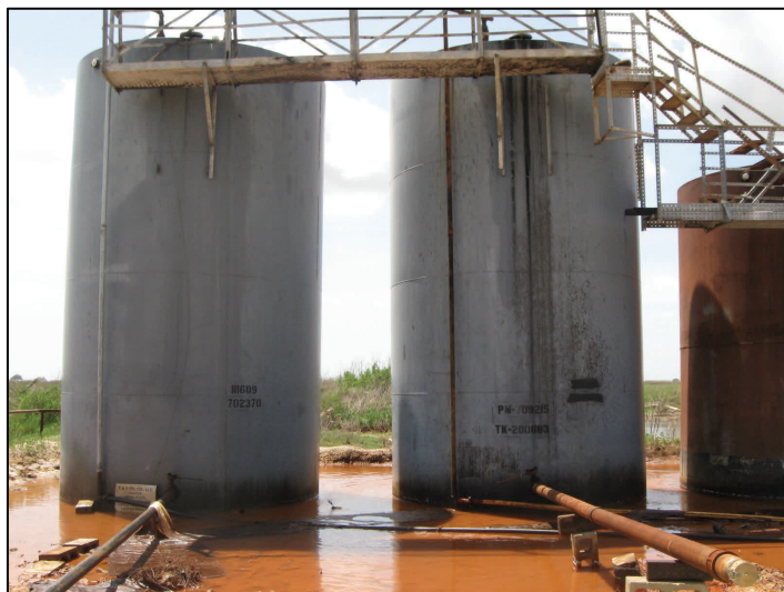
Oil pooled around T & F storage tanks
