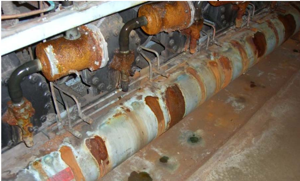
Figure 2: Excessive corrosion on rack components
