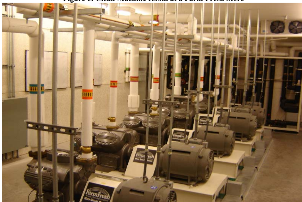
Figure 6: Clean Machine Room at a Farm Fresh Store
