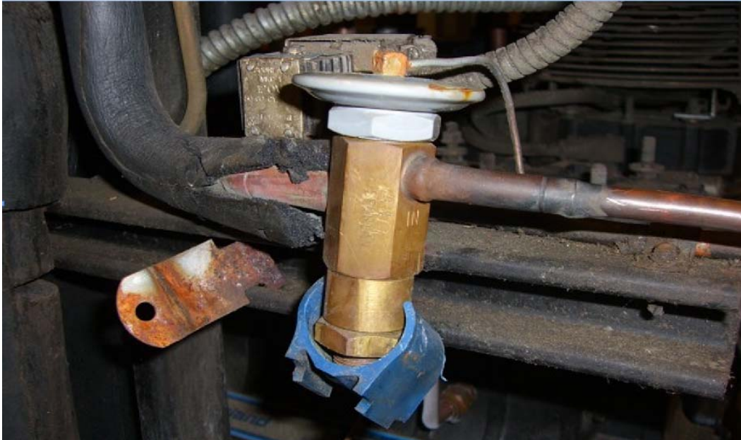
Figure 4: Image of broken clamp caused by vibrations
