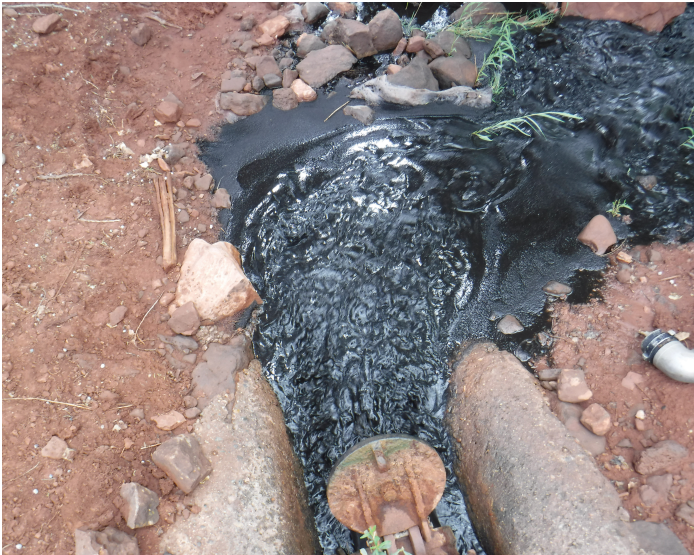
Fig 1: Manganese contaminants leaving a water system following ice pigging.
