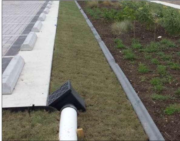
Figure 2. Finished bioswale at Cascade Park.
