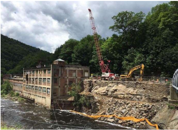
Cleanup in progress, along edge of river (photo credit Franklin Regional Council of Governments)
