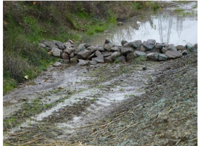
A rock check dam in a channel. Credit: Kort Kirkeby for USEPA, 2012
