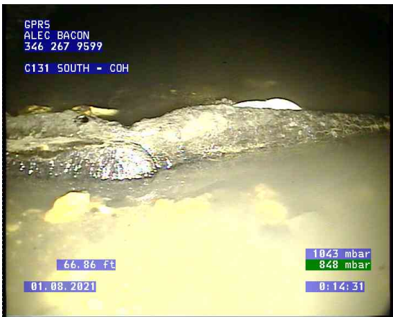
C131 SOUTH - COH_0003.bmp, , 66.86ft Deformed Horizontal, 5% changed
