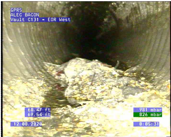
Vault C131 - EOR West_0008.bmp, , 68.50ft Obstacles Other, 5% of cross sectional area at 6 o'clock / debris
