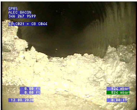
CB C021 - CB C044_0002.bmp, , 0.00ft Deposits Settled Compacted, 40% of cross sectional area from 3 o'clock to 9 o'clock
