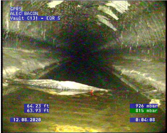
Vault C131 - EOR S_0004.bmp, , 64.24ft Obstacles Other, 5% of cross sectional area at 7 o'clock / unknown
