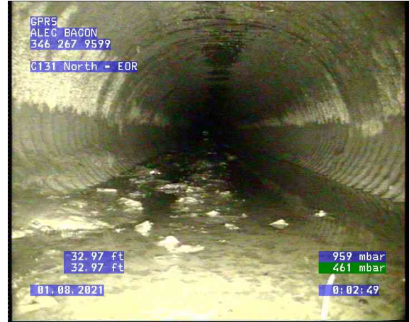
C131 North - EOR_0001.bmp, , 32.97ft Deposits Settled Gravel, 5% of cross sectional area from 4 o'clock to 8 o'clock, Start
