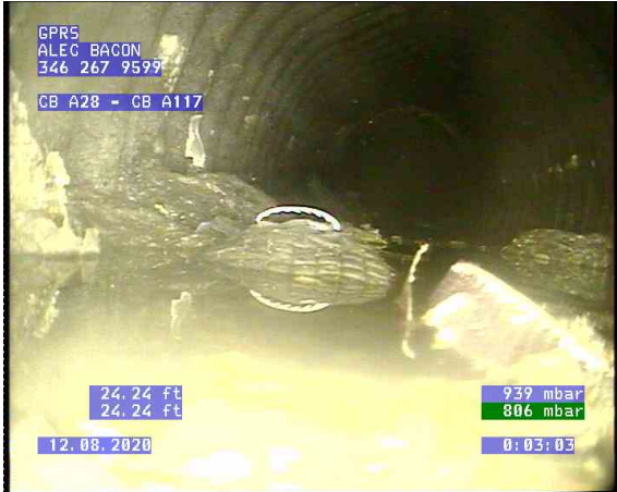
CB A28 - CB A117_0002.bmp, , 24.25ft Survey Abandoned / could not make it past deposit
