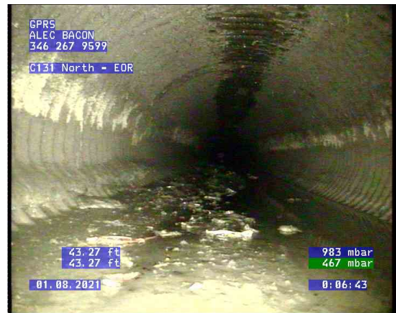
C131 North - EOR_0003.bmp, , 43.27ft Survey Abandoned / stuck in mud
