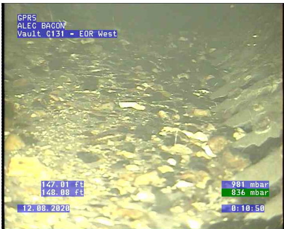
Vault C131 - EOR West_0014.bmp, , 147.05ft Deformed Horizontal, 5% changed, Finish
