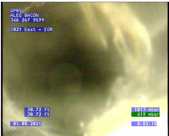
C021 East - EOR_0002.bmp, , 30.74ft Roots Medium Joint from 1 o'clock to 5 o'clock, 5% lost
