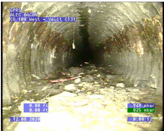
CB C108 West - Vault C131_0002.bmp, , 0.00ft Water Level
