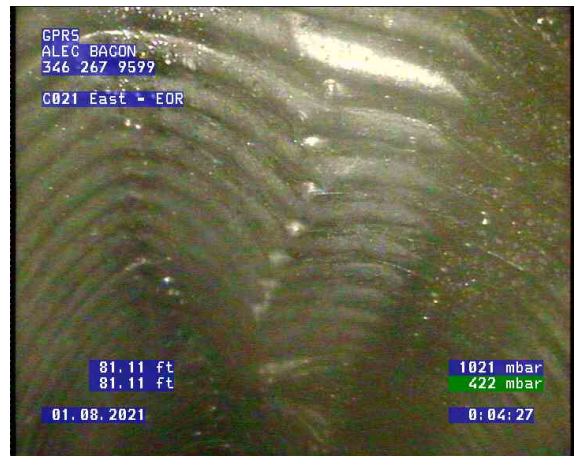
C021 East - EOR_0003.bmp, , 81.14ft Deformed, 10% changed, Start
