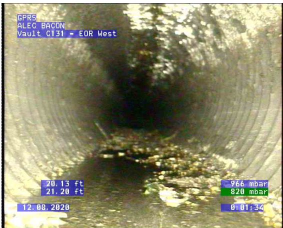
Vault C131 - EOR West_0002.bmp, , 20.14ft Deposits Settled Gravel, 10% of cross sectional area from 5 o'clock, Start
