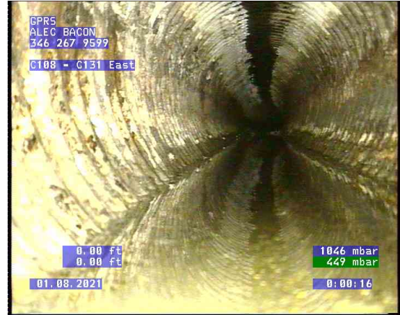
C108 - C131 East_0001.bmp, , 0.01ft Surface Corrosion Metal Pipe from 12 o'clock to 11 o'clock, Start
