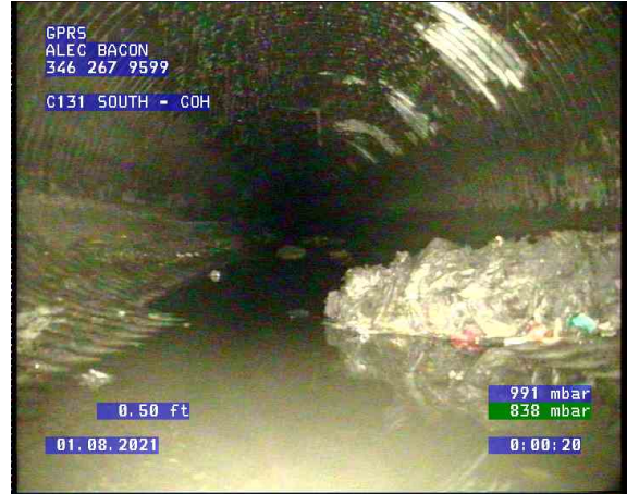
C131 SOUTH - COH_0001.bmp, , 0.49ft Deposits Settled Compacted, 10% of cross sectional area from 4 o'clock to 6 o'clock
