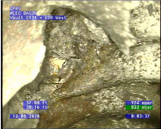
Vault C131 - EOR West_0004.bmp, , 37.11ft Deformed, 5% changed
