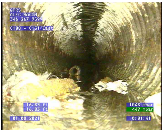
C108 - C131 East_0002.bmp, , 16.83ft Obstacles Other, 10% of cross sectional area from 4 o'clock to 8 o'clock / debris
