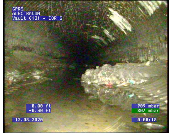
Vault C131 - EOR S_0002.bmp, , 0.00ft Deposits Settled Compacted, 10% of cross sectional area at 4 o'clock
