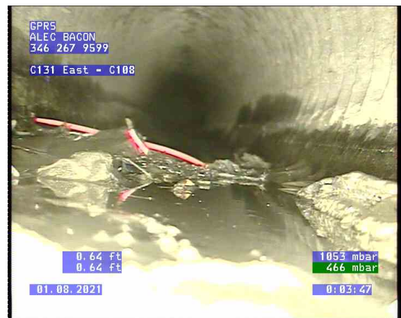
C131 East - C108_0003.bmp, , 0.62ft Surface Corrosion Metal Pipe from 12 o'clock to 11 o'clock, Finish
