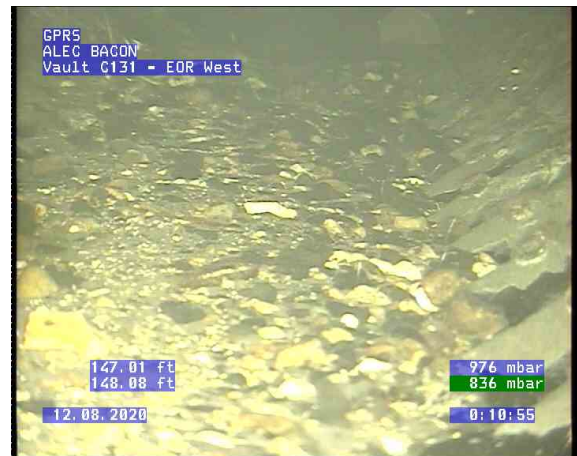
Vault C131 - EOR West_0015.bmp, , 147.05ft Camera Underwater
