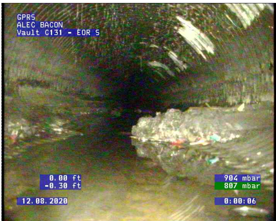
Vault C131 - EOR S_0000.bmp, , 0.00ft Junction Box / vault
