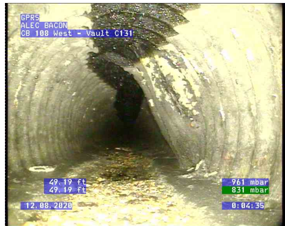
CB C108 West - Vault C131_0003.bmp, , 49.21ft Collapse Pipe Sewer, 45% lost
