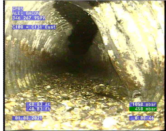
C108 - C131 East_0005.bmp, , 48.85ft Deformed, 20% changed
