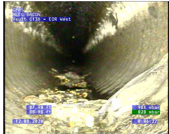
Vault C131 - EOR West_0009.bmp, , 87.93ft Obstacles Other, 5% of cross sectional area at 6 o'clock / debris
