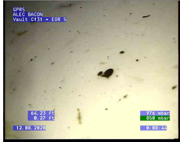
Vault C131 - EOR S_0005.bmp, , 64.24ft Obstacles Other, 5% of cross sectional area at 7 o'clock / unknown
