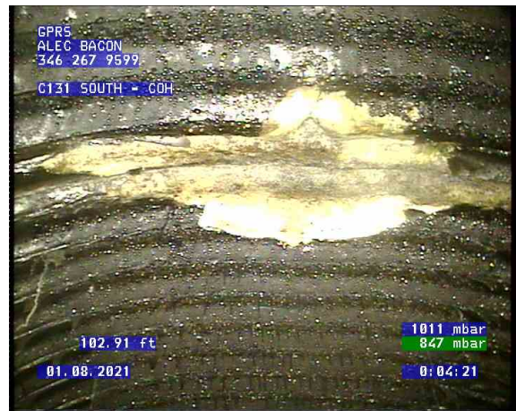
C131 SOUTH - COH_0002.bmp, , 102.95ft Surface Missing Wall Unknown at 12 o'clock
