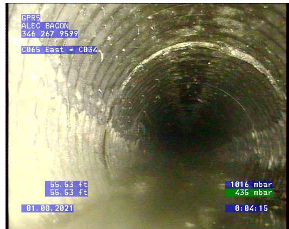
C065 East - C034_0003.bmp, , 55.54ft Survey Abandoned / stuck in mud
