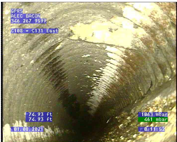
C108 - C131 East_0006.bmp, , 74.97ft Deformed, 5% changed
