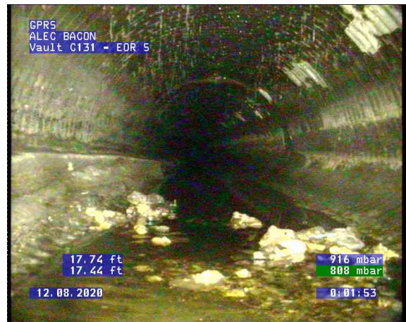
Vault C131 - EOR S_0003.bmp, , 17.75ft Obstacles Rocks, 5% of cross sectional area from 5 o'clock to 7 o'clock
