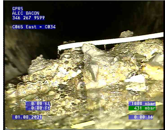
C065 East - C034_0001.bmp, , 0.00ft Deposits Settled Other, 10% of cross sectional area from 4 o'clock to 8 o'clock / rocks and more
