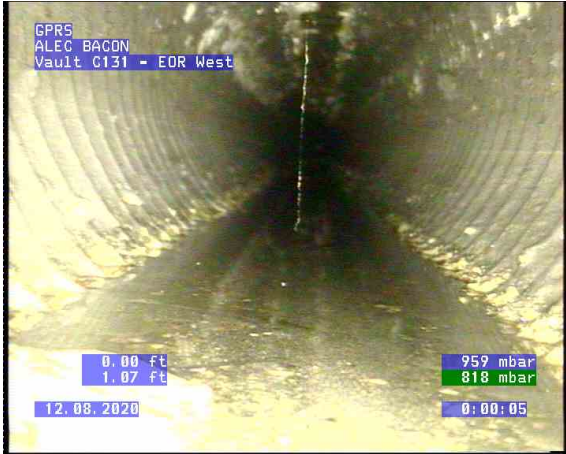
Vault C131 - EOR West_0000.bmp, , 0.00ft Junction Box / vault
