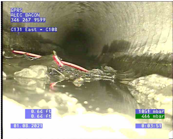
C131 East - C108_0004.bmp, , 0.66ft Survey Abandoned / stuck in mud
