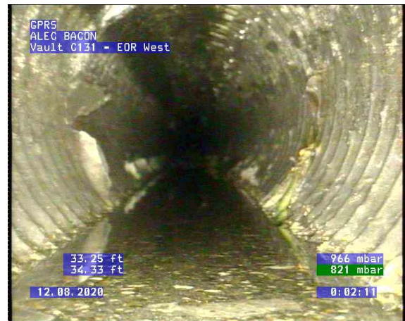
Vault C131 - EOR West_0003.bmp, , 33.27ft Deposits Settled Gravel, 10% of cross sectional area from 5 o'clock, Finish
