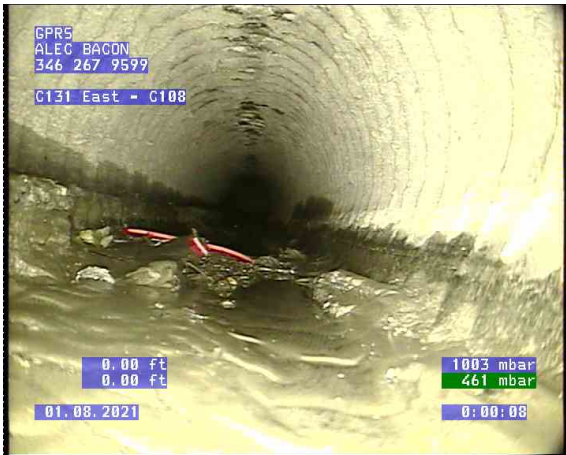
C131 East - C108_0001.bmp, , 0.00ft Deposits Settled Compacted, 15% of cross sectional area from 4 o'clock to 8 o'clock, Start
