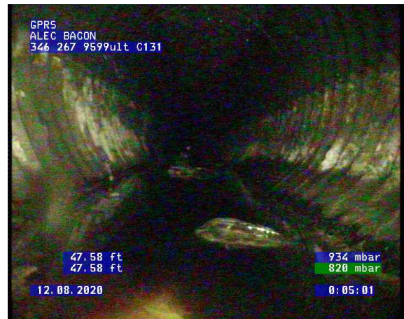
CB C065 - Vault C131_0003.bmp, , 47.61ft Deposits Settled Compacted, 10% of cross sectional area from 5 o'clock to 7 o'clock, Finish
