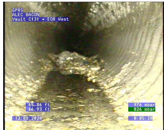
Vault C131 - EOR West_0007.bmp, , 65.88ft Deposits Settled Gravel, 5% of cross sectional area from 5 o'clock, Finish
