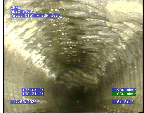
Vault C131 - EOR West_0013.bmp, , 137.66ft Deformed Horizontal, 5% changed, Start
