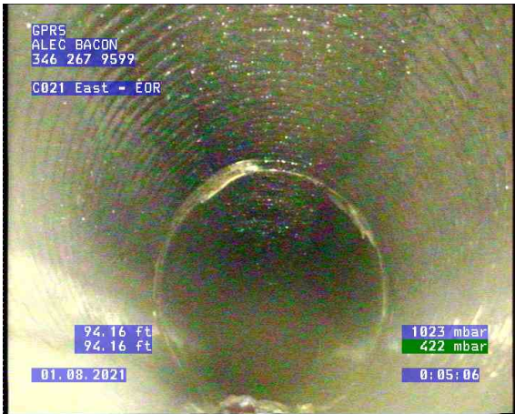
C021 East - EOR_0004.bmp, , 94.19ft Deformed, 10% changed, Finish
