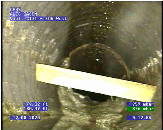
Vault C131 - EOR West_0016.bmp, , 179.36ft Obstacles External Pipe or Cable, 20% of cross sectional area from 4 o'clock to 9 o'clock
