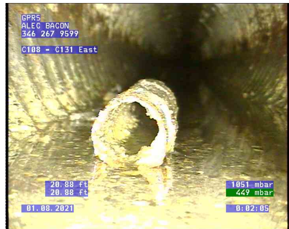
C108 - C131 East_0003.bmp, , 20.90ft Obstacles Other, 10% of cross sectional area at 7 o'clock / debris
