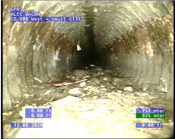
CB C108 West - Vault C131_0000.bmp, , 0.00ft Deposits Settled Compacted, 15% of cross sectional area from 5 o'clock to 7 o'clock, Start
