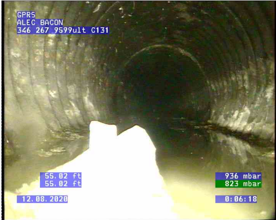
CB C065 - Vault C131_0004.bmp, , 55.02ft Survey Abandoned / could not make it past deposit
