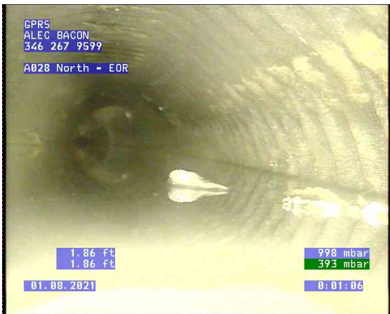
A028 North - EOR_0002.bmp, , 1.87ft Survey Abandoned / stuck in mud
