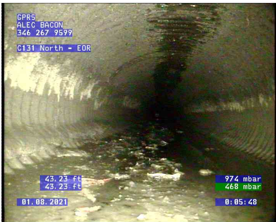
C131 North - EOR_0002.bmp, , 43.24ft Deposits Settled Gravel, 5% of cross sectional area from 4 o'clock to 8 o'clock, Finish
