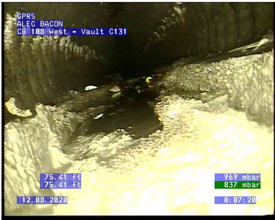
CB C108 West - Vault C131_0004.bmp , 75.43ft Survey Abandoned / could not drive through deposit
