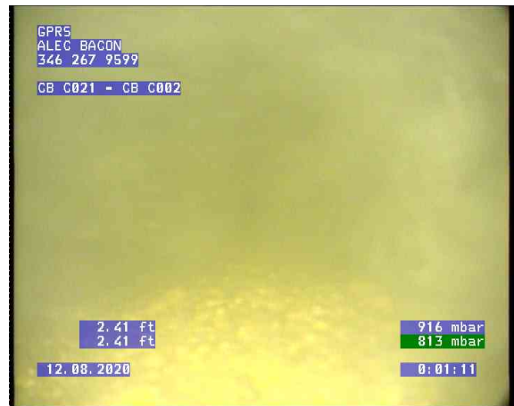
CB C021 - CB C002_0003.bmp, , 2.40ft Survey Abandoned / camera underwater
