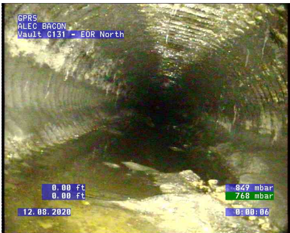
Vault C131 - EOR North_0000.bmp, , 0.00ft Junction Box / vault
