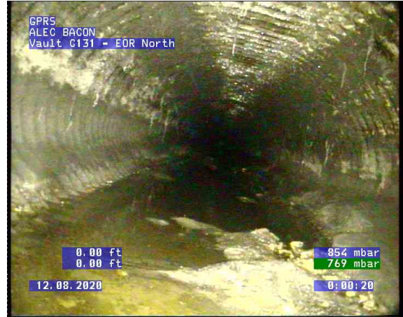
Vault C131 - EOR North_0002.bmp, , 0.00ft Deposits Settled Compacted, 5% of cross sectional area at 5 o'clock
