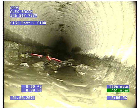
C131 East - C108_0002.bmp, , 0.00ft Surface Corrosion Metal Pipe from 12 o'clock to 11 o'clock, Start
