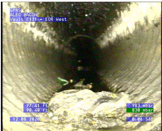
Vault C131 - EOR West_0010.bmp, , 97.44ft Obstacles Other, 5% of cross sectional area at 6 o'clock / debris
