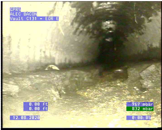
Vault C131 - EOR E_0000.bmp, , 0.00ft Junction Box / vault
