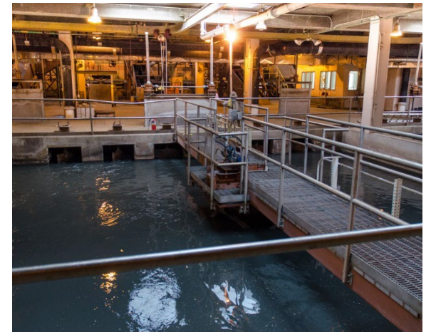
Treatment plants needed repairs after Hurricane Sandy (EPA)
