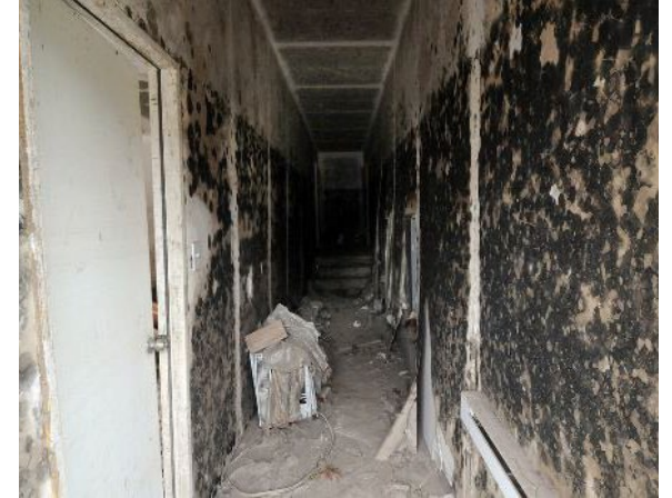
Moldy walls after Hurricane Sandy (FEMA)
