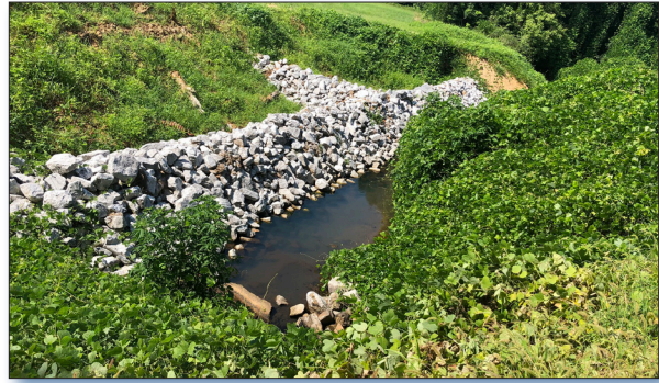
Figure 4. Streambank and shoreline protection BMP.
