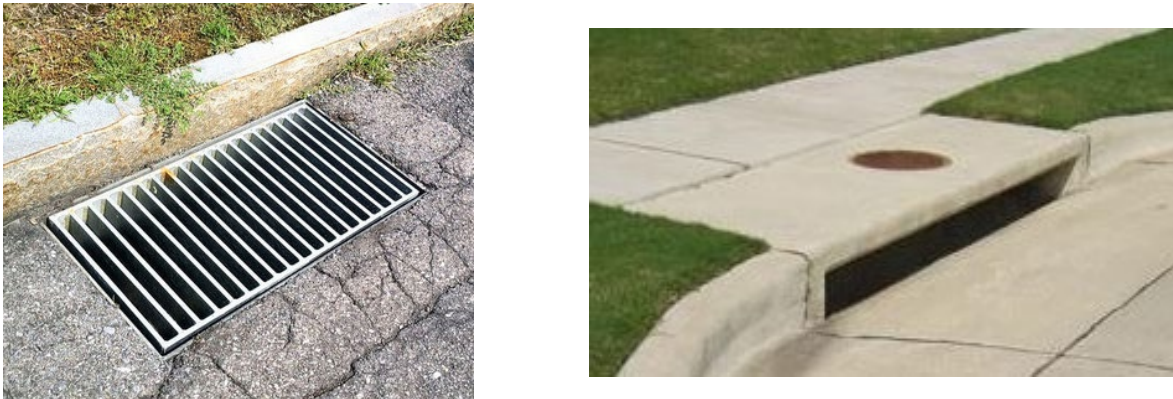
Figure 4. Examples of storm drain inlets.
