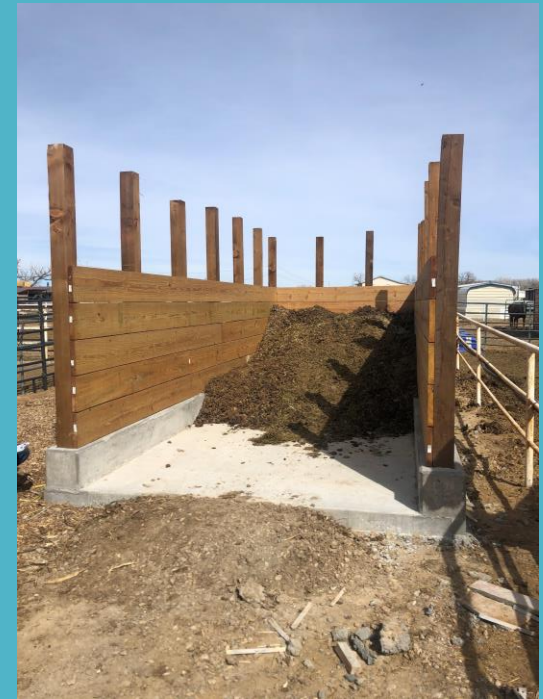
2020 Four Corners Equine Rescue Waste Containment Facilities
