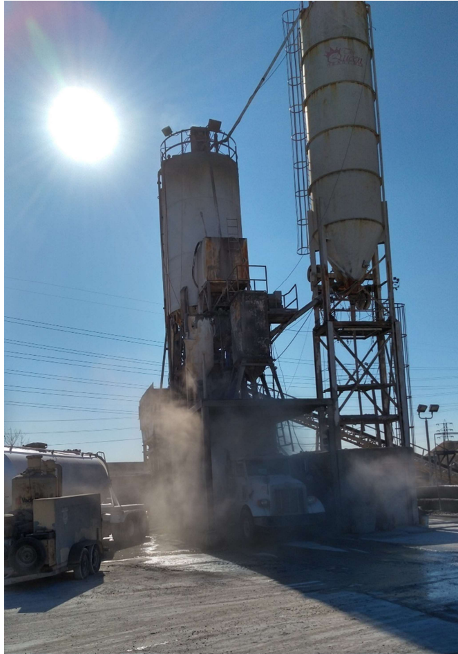
View of regular loading operations at the baghouse
