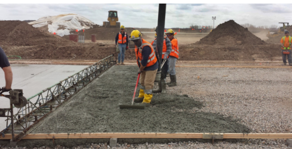
Workers lay foundation for the new 700-megawatt natural gas-fueled power generation facility constructed by Competitive Power Ventures.
