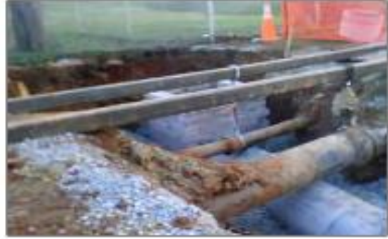
Repair of City of Mebane Sewer and Water lines leaking into Stream at City Park (Feb. 2007)
