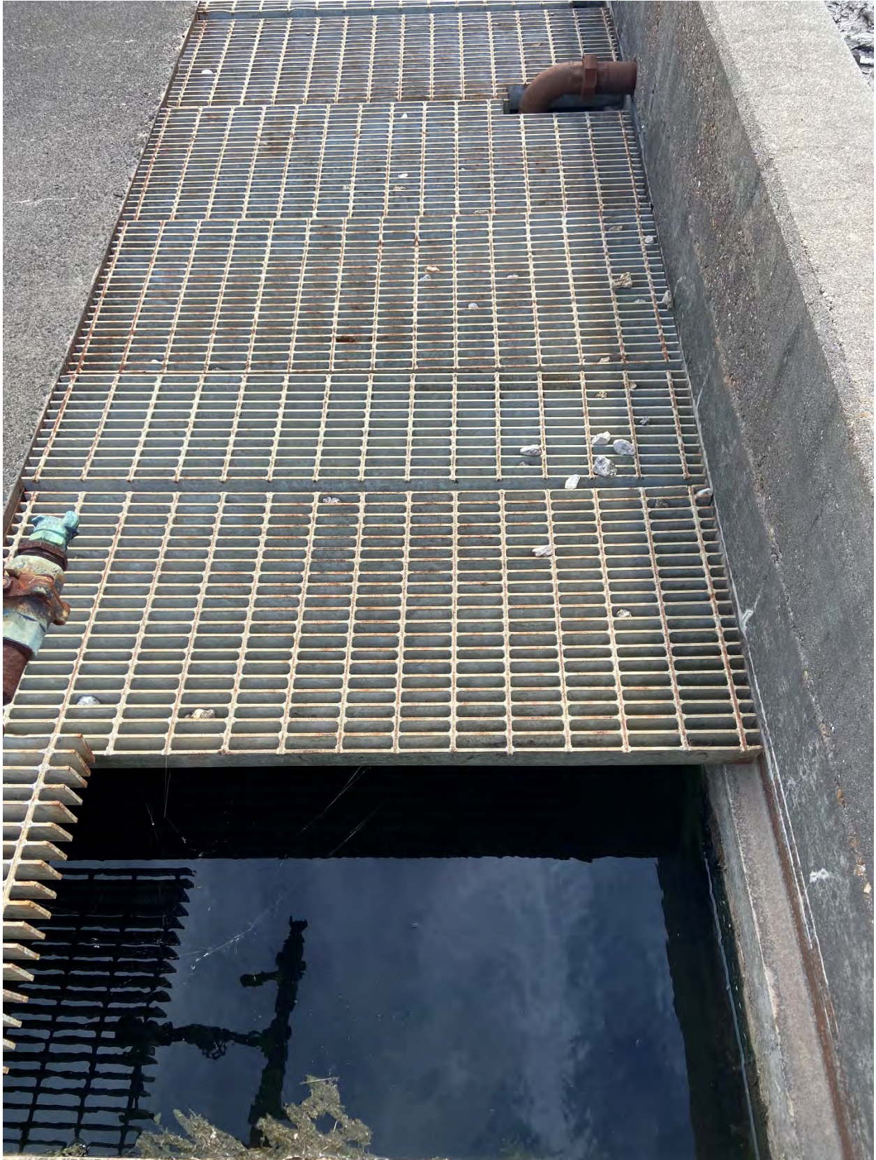
SWMU-5 Slop Oil Sump
