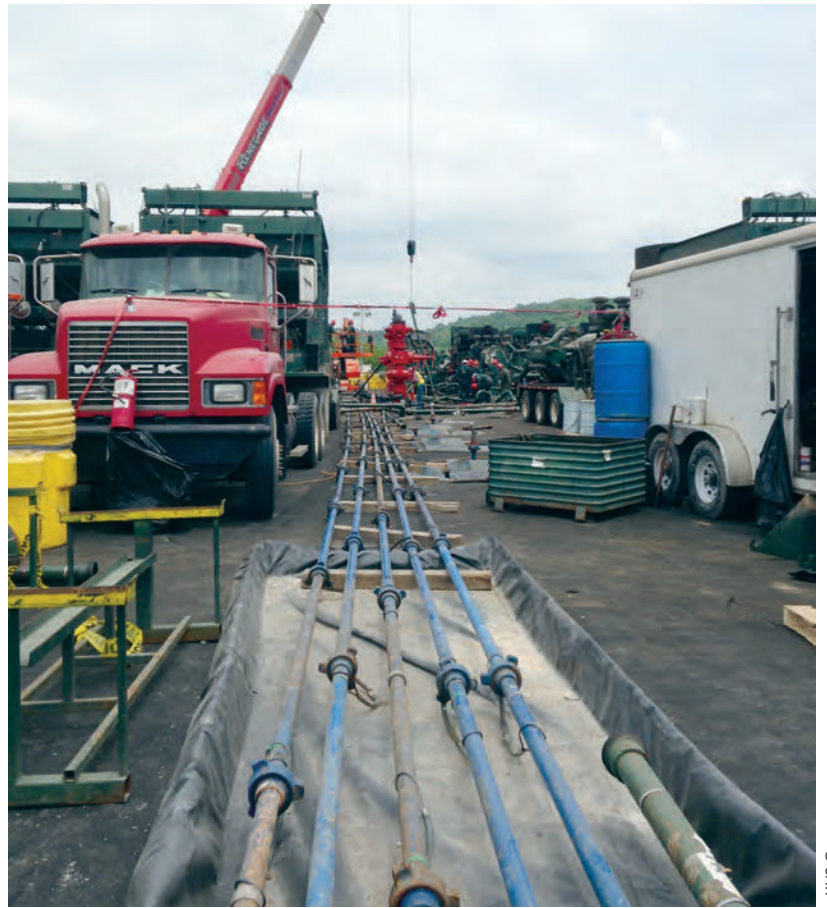
Completion equipment at a gas well.
