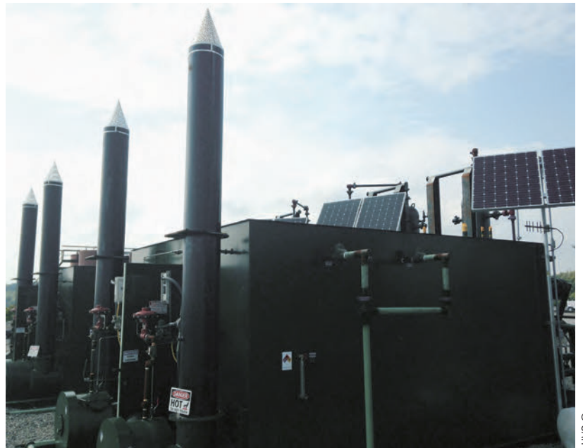
Equipment at a gas well.
