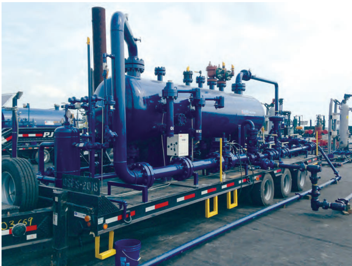
Equipment at a gas well.
