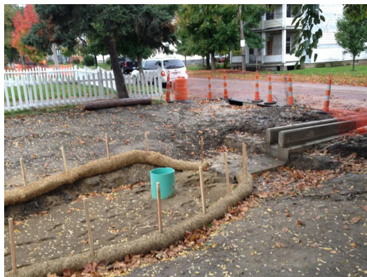
A NEORSD vacant lot during the construction process. Courtesy of the Northeast Ohio Regional Sewer District.
