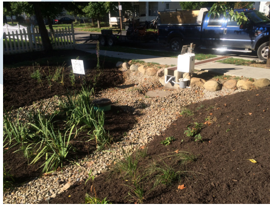
One of the completed NEORSD bioretention features. Courtesy of the Northeast Ohio Regional Sewer District.
