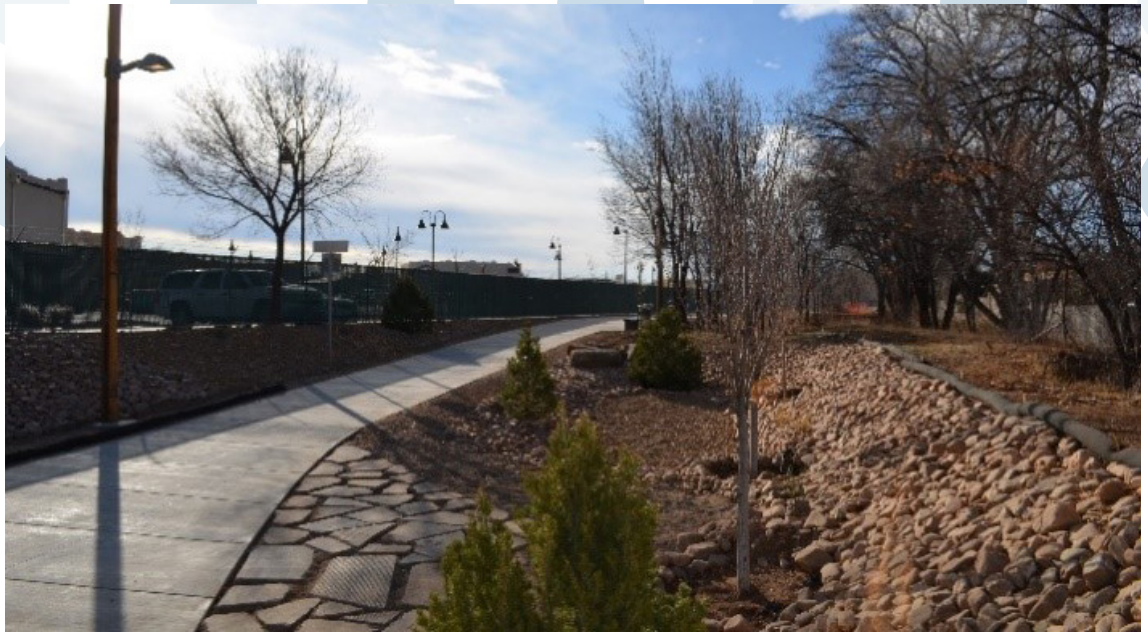
A bioswale constructed from gravel and repurposed concrete reduces erosion and directs stormwater flow. Courtesy Serquis + Associates
