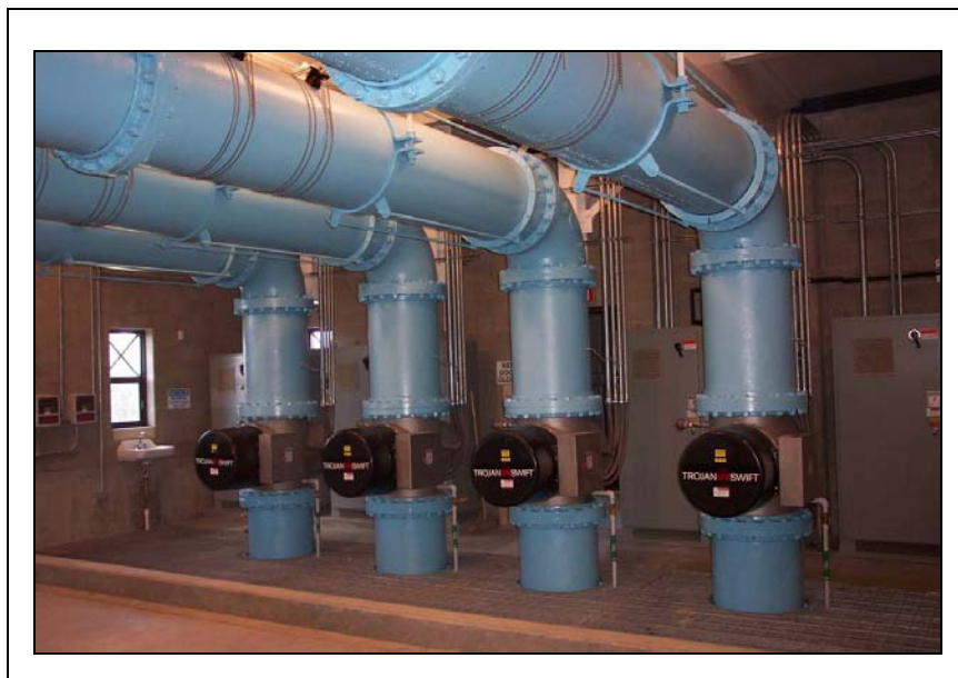
Figure F.5. UV Disinfection Facility at the Loudonville Reservoir
