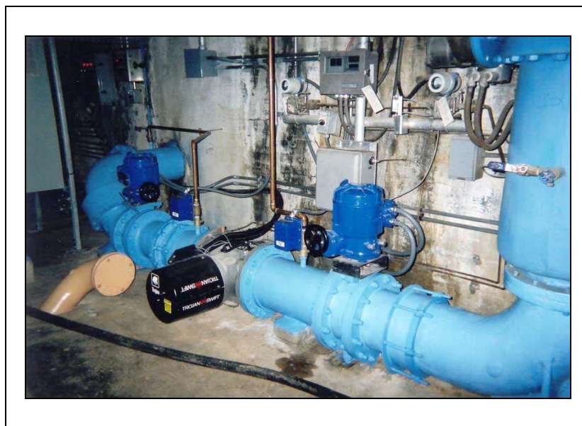
Figure F.15. UV Reactor at the Newark WTP
