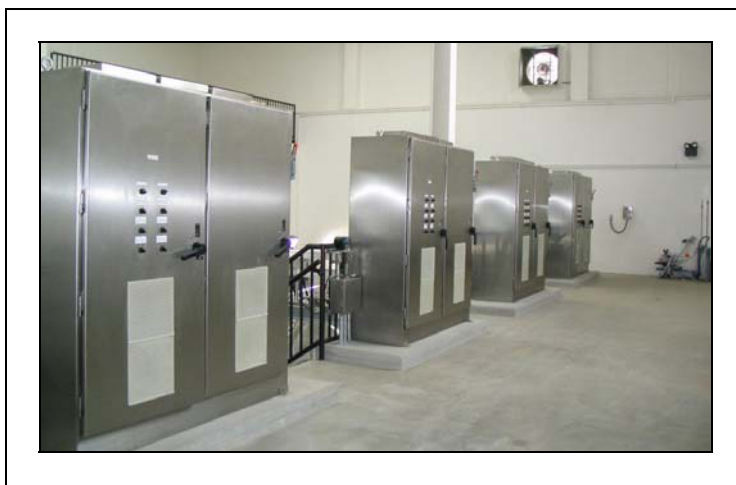
Figure F.14. UV Reactor Electrical Cabinets at the Weber WTP No. 3 (the floor above the UV reactors)
