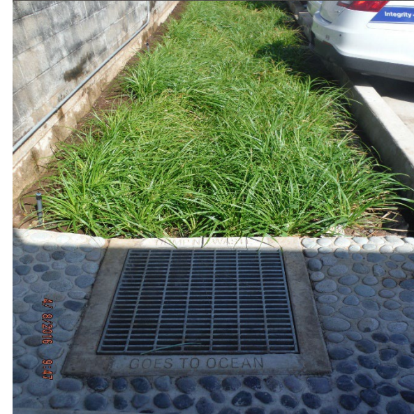
Biofiltration Swale at HPD Police Station
