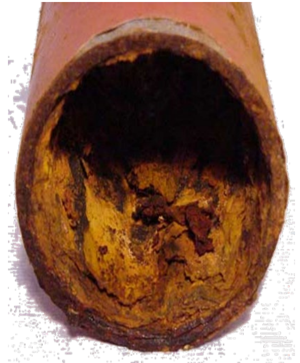
Rusted iron water pipe
