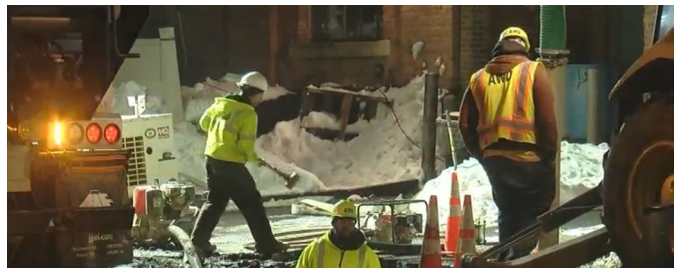
Many water utilities use GPS to locate valves more quickly when responding to water main breaks.
