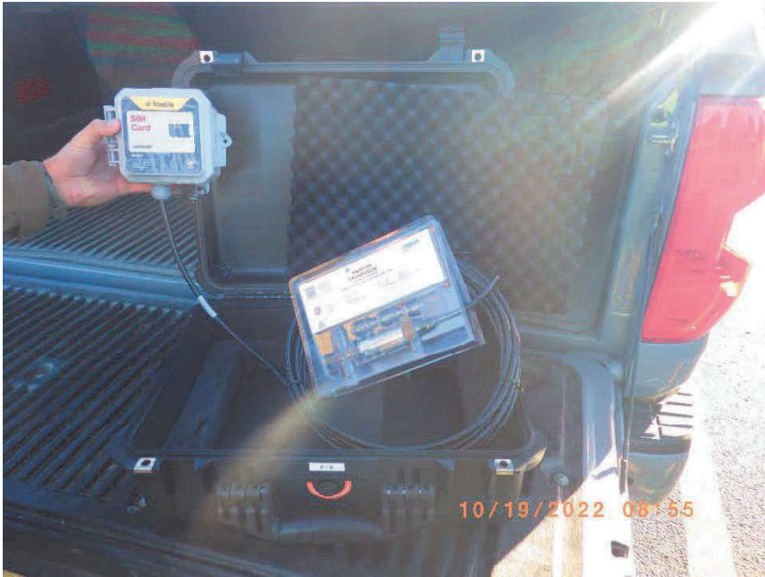
14: RIMG1614 Description: Pressure Monitoring Equipment Location: Illinois American Warehouse Date/Time: 10-19-2022
