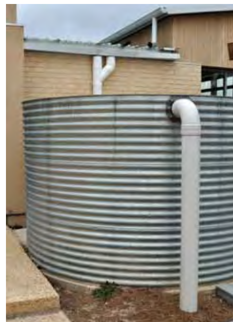
Rainwater collection system
