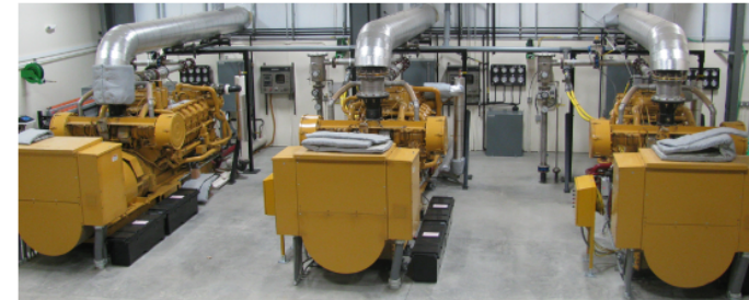
LFG-fired engines at Western Regional Landfill, California. Used with permission from Energy 2001.
