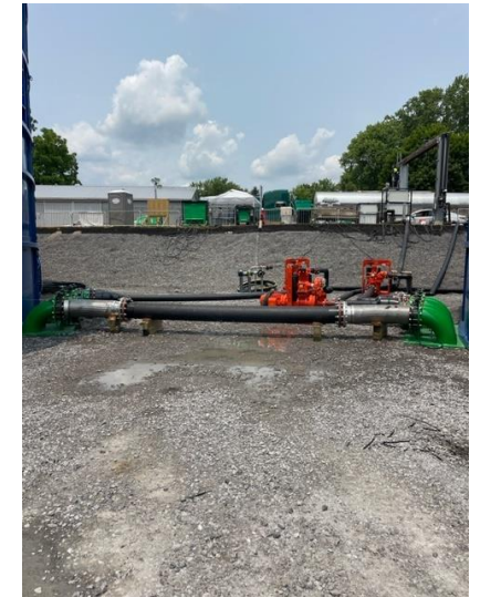
Manifolding between Tanks
