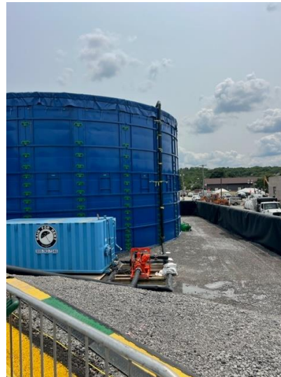
Tank #2 West Fill line
