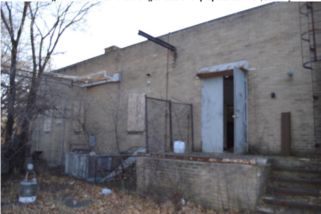
Photo 3 Detail of loading dock area and north wall proposed for demolition, January 2023
