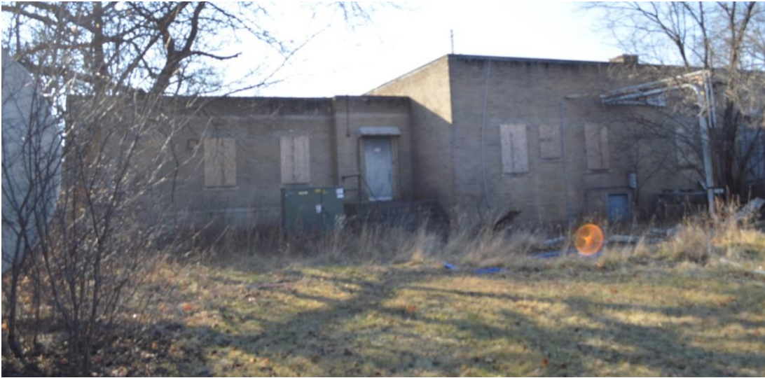
Photo 4 Looking south at area for proposed barrier free ramp and north wall where addition is proposed, January 2023
