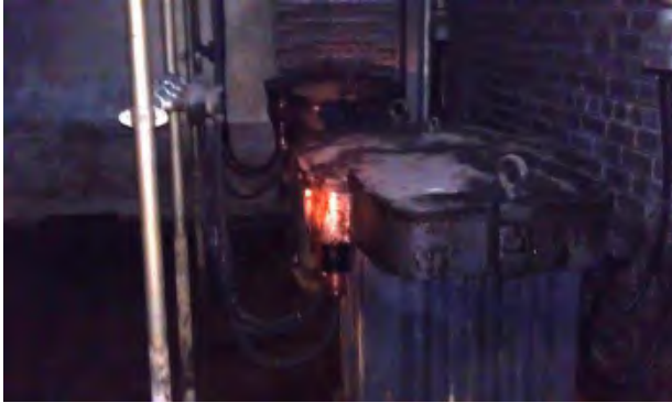
Photo #1 View of Transformers in the Basement.
