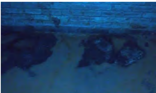
Photo #5 View of tar like material below the Pot Heads.
