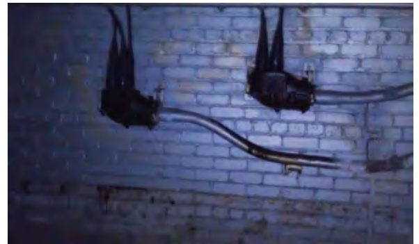
Photo #4 View Pot Heads on the basement wall.
