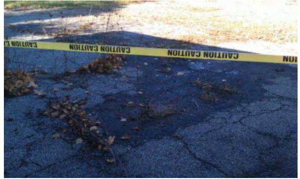
Photo #8 View oil stained pavement outside of the garage.
