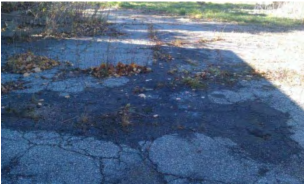
Photo #9 View oil stained pavement outside of the garage.
