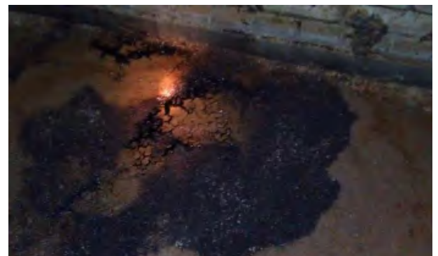
Photo #6 View of tar like material below the Pot Heads.
