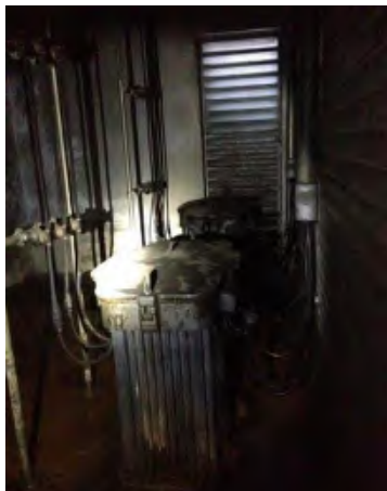
Photo #3 View of Transformers in the Basement.
