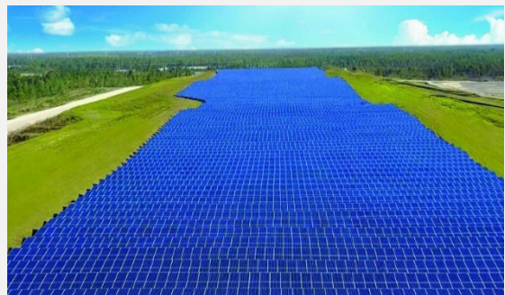
OUC’s Community Solar Plant. Photo courtesy of Orlando Utility Commission
