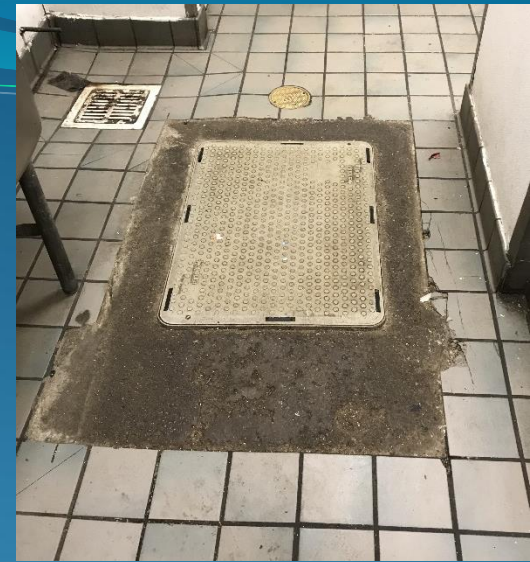
In Floor Grease Trap
