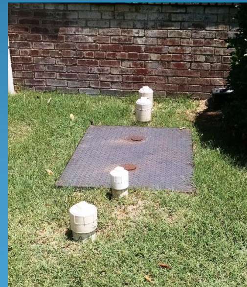
Outside, in-ground Grease Trap
