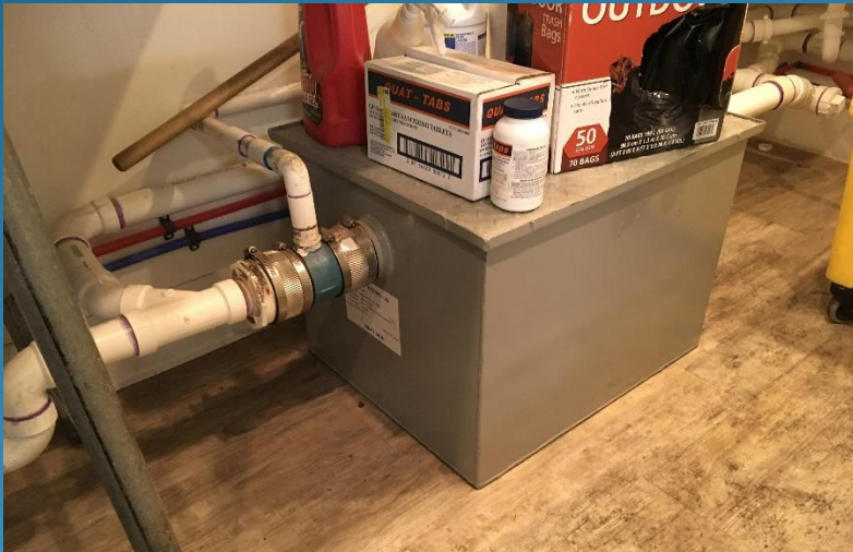
Under the Sink Grease Trap
