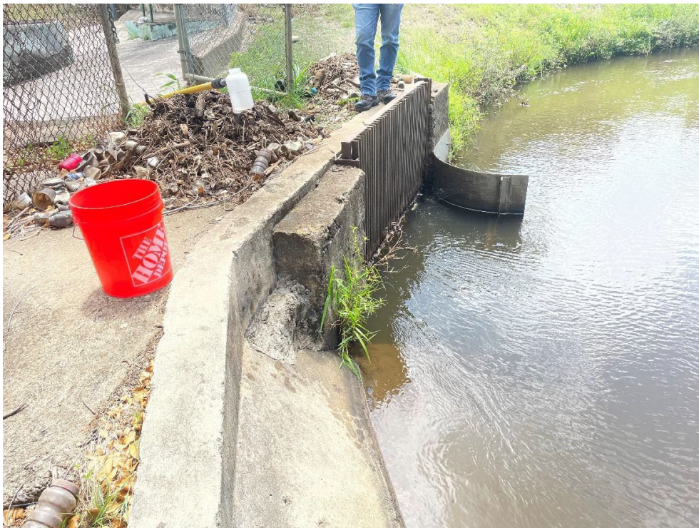
Photograph 8: View of the bar screen in the irrigation channel that screens raw water prior to its entrance into the pump station.
