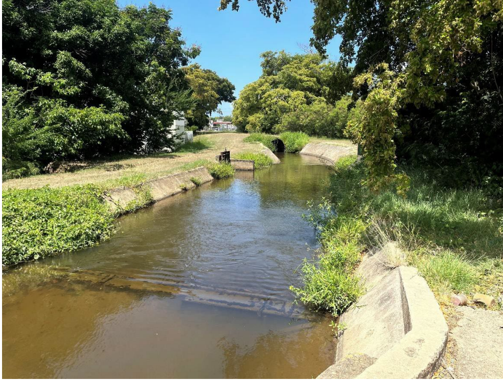
Photograph 7: View of the irrigation channel after the intake location. Raw water comes from Patillas Lake located northeast and continues after the intake of the Rexmanor Pump Station to the west.
