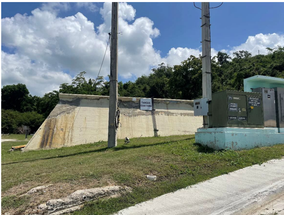
Photograph 4: View of the Guayama DWTP 250,000-gallon tank for storage and distribution of treated water.
