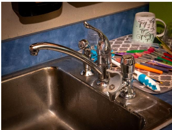
The image above is of a Classroom Faucet (CF) and Drinking Water Fountain (DW) that were sampled at a school. There were multiple schools with two (2) fixtures on each sink. These are often found in schools built prior to 1980.
