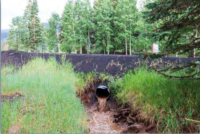
Culvert of lower drainage system flowing into previously eroded gully on Hart Prairie, July 18, 2021 around 4 pm. Culvert passes under Forest Road 516. Culvert was well over half-full in the surge of the first of two runoff events. The second surge was almost half-full, which is above the level in the photograph.
