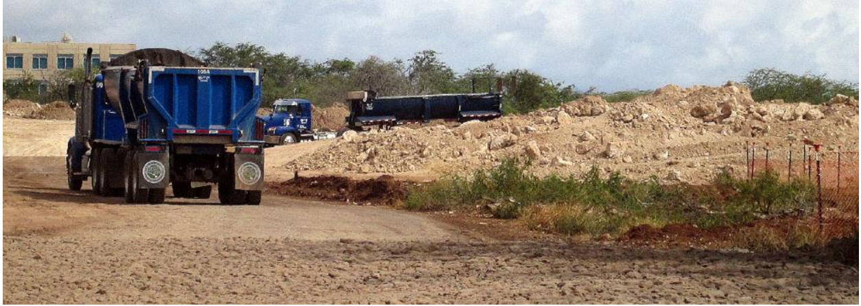
The scale of the Hunt contaminated soil dumping on Parcel 12 has grown massively over several months
