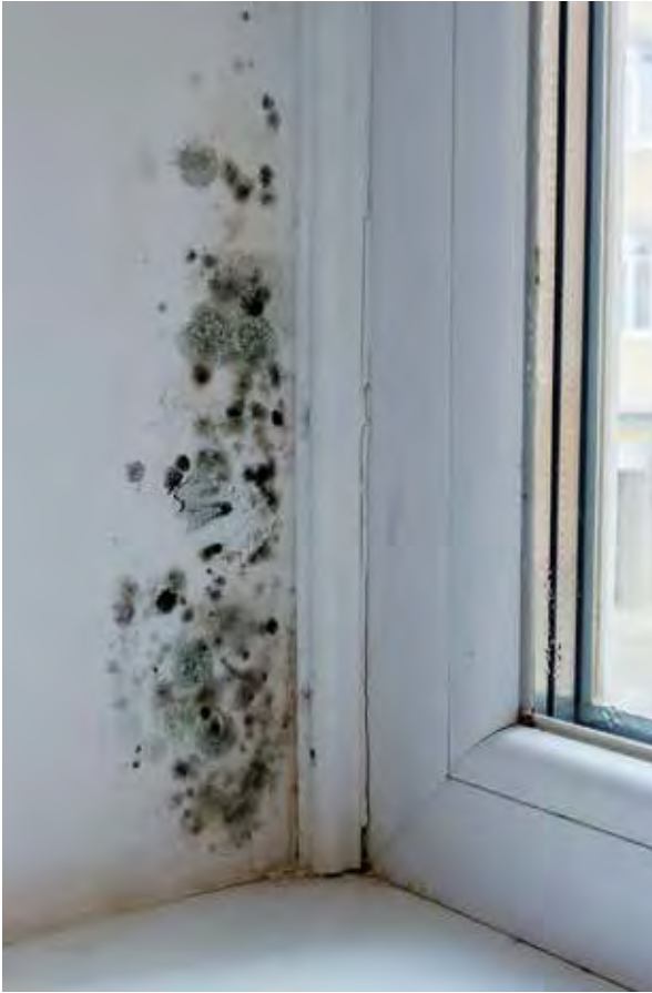
The combination of higher temperatures and increased precipitation can lead to increased mold production in buildings and negative impacts to human health.
