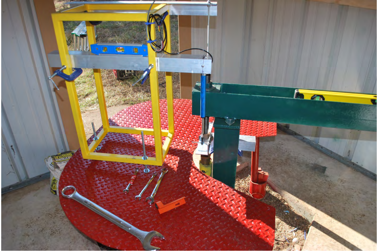
Figure 3. Installation of new equipment and a digital potentiometer on the Suffolk extensometer (58C 52). Photograph by David Nelms, February 18, 2016.
