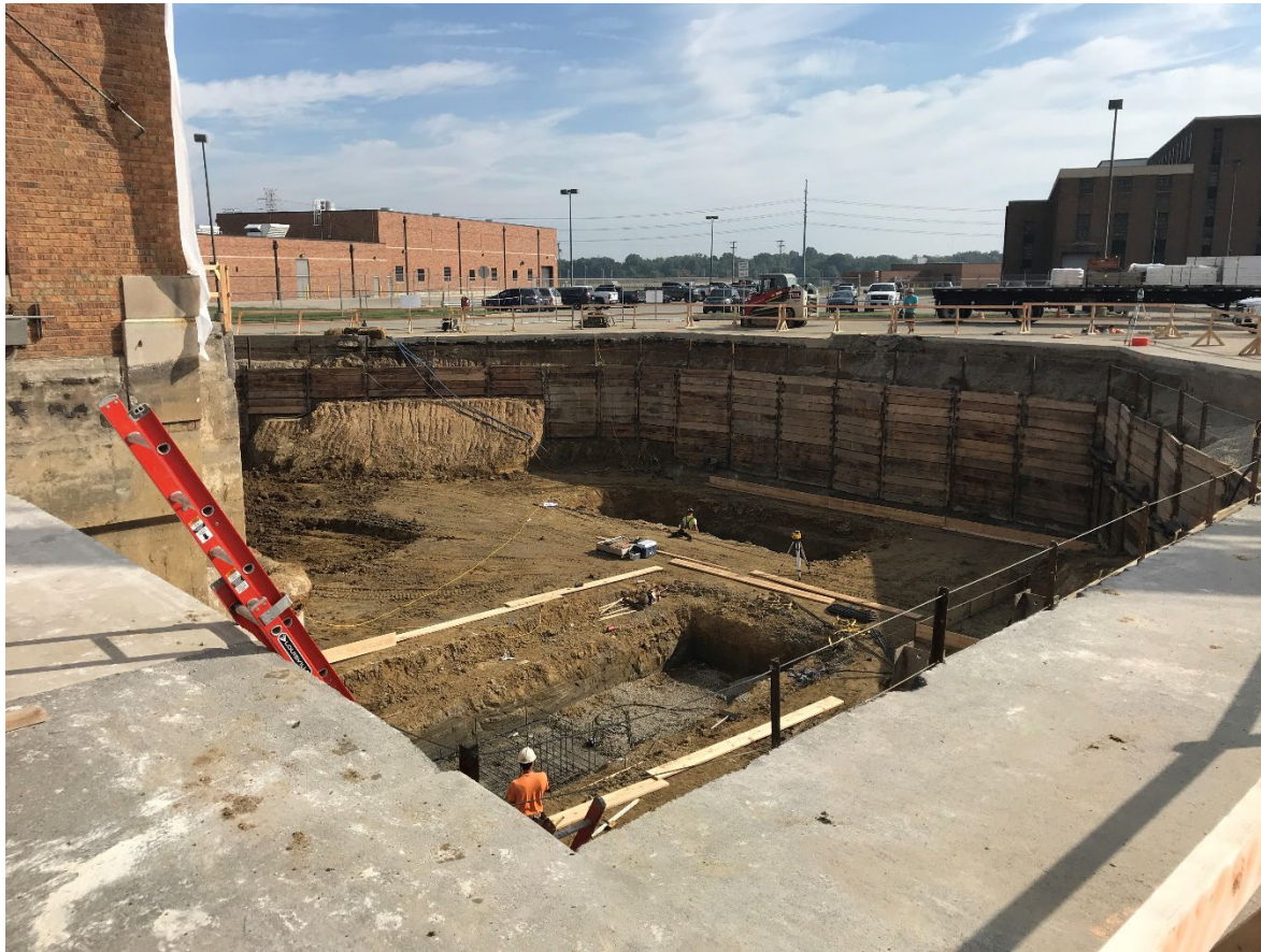
Water Plant Springfield, Illinois
