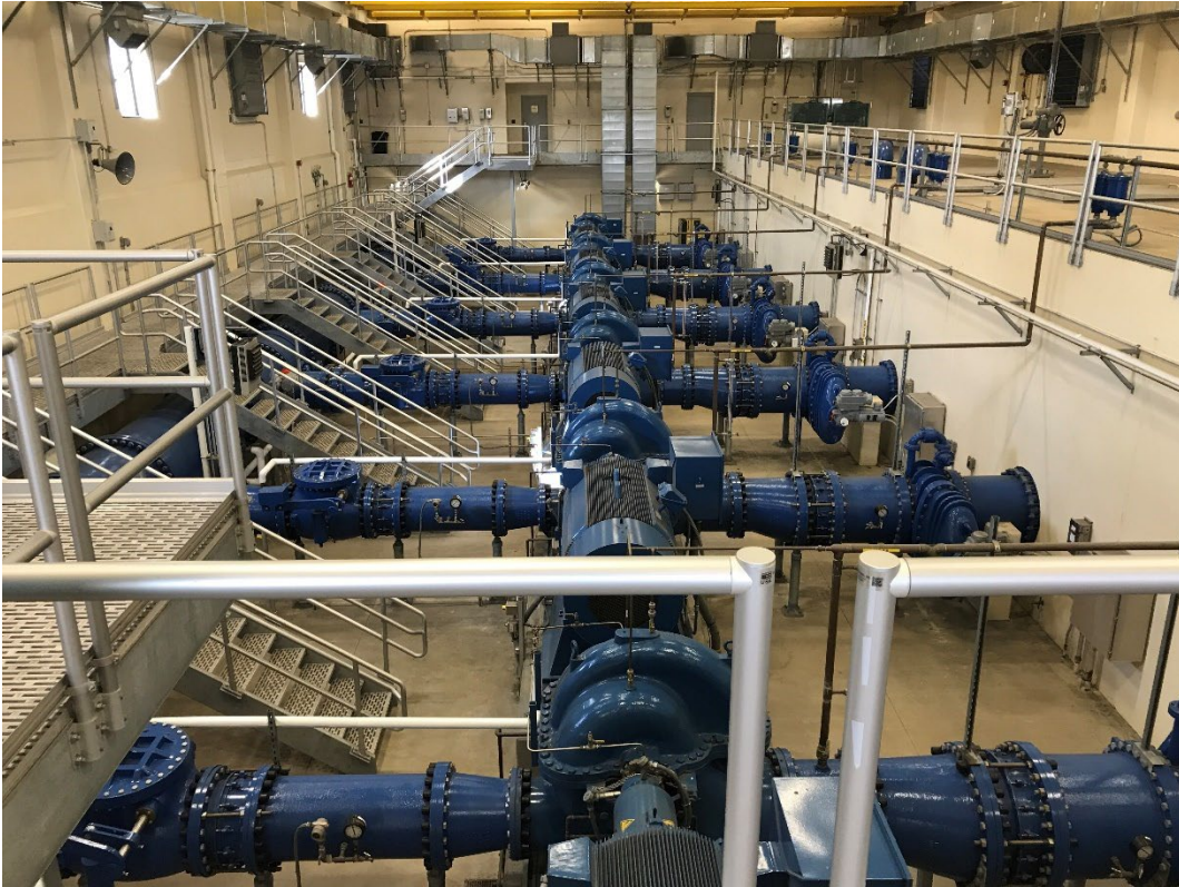
Water Plant Springfield, Illinois
