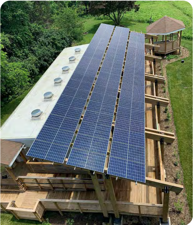
Solar array at M-NCPPC’s Maydale Conservation Park
