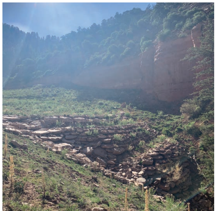
Mesa II in May 2022, four years after a time critical removal action was conducted on site in 2018 by US EPA.
