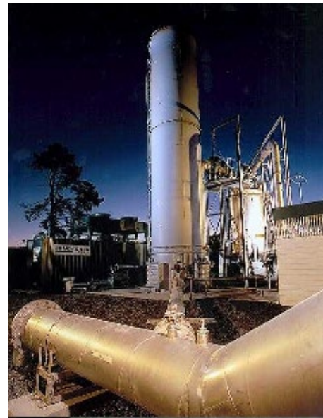
Figure 3-10. Submerged Combustion Leachate Evaporator
