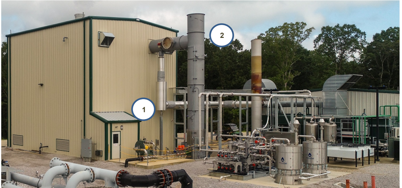
Figure 3-12. Concentrator Type of Leachate Evaporator – Heartland’s Low Momentum-High Turbulence (LM-HT®) Evaporator Using Heat from Both (1) Engine Exhaust and (2) LFG Flare
