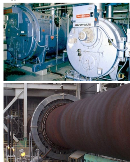
Figure 3-6. Boiler and Cement Kiln
