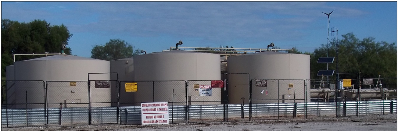
Figure 3-3. Liquid Storage Tanks
