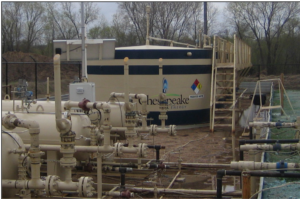
Figure 3-15. Produced Water Tanks
