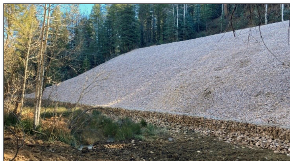
Figure 4. Regraded and capped waste pile with new gabion wall at the toe.
