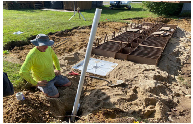
Installation of a denitrifying Fujiclean septic system to a pressurized GST™ drainfield. A pan lysimeter was installed beneath the GST™ forms to allow for the collection and monitoring of post soil treatment area effluent for comparative analysis between various soil treatment area types. Photo credit: Matthew Dowling
