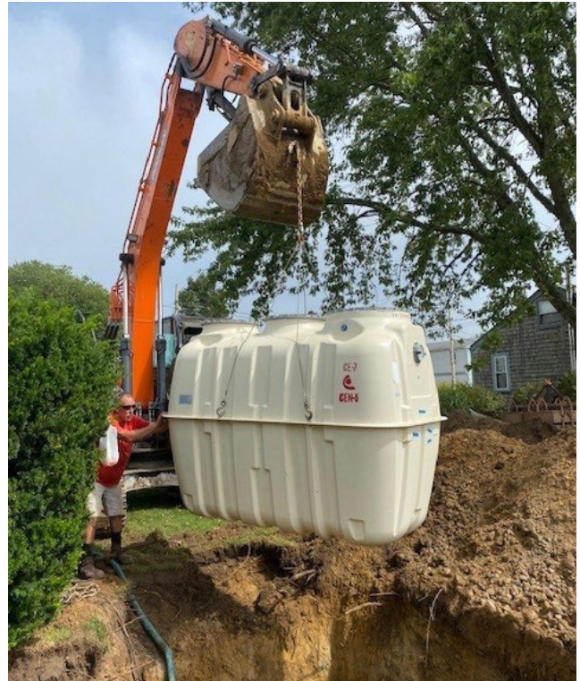
Installation of a Fujiclean denitrifying OWTS to replace a failing conventional septic system. Photo credit: Matthew Dowling
