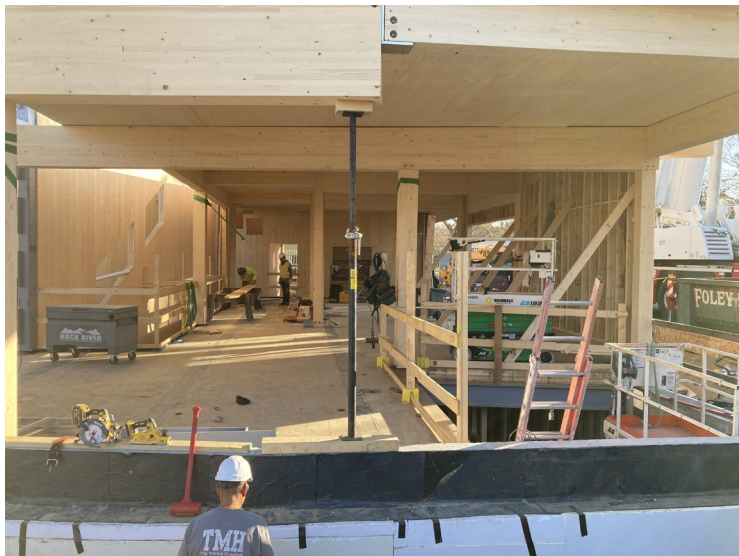
The new Community MusicWorks Center in Providence taking shape. SWIG funded water management features and plantings on the site that will minimize stormwater runoff while contributing to climate resilience in this environmental justice neighborhood. The building itself is built from cross-laminated timber panels – a high-tech wood construction method that is carbon neutral, while providing excellent acoustics. Photo credit: Restore America's Estuaries
