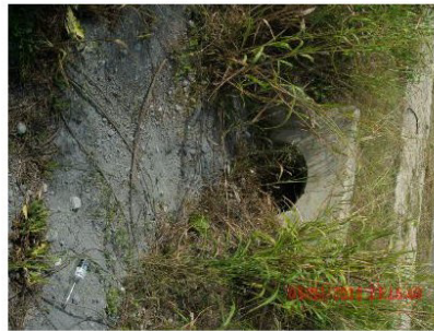
Coal ash in storm water sewer system
