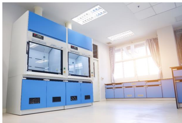
Laboratory fume hoods
