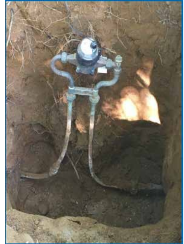
Example of Meter Pit Source LSLR Collaborative 2018
